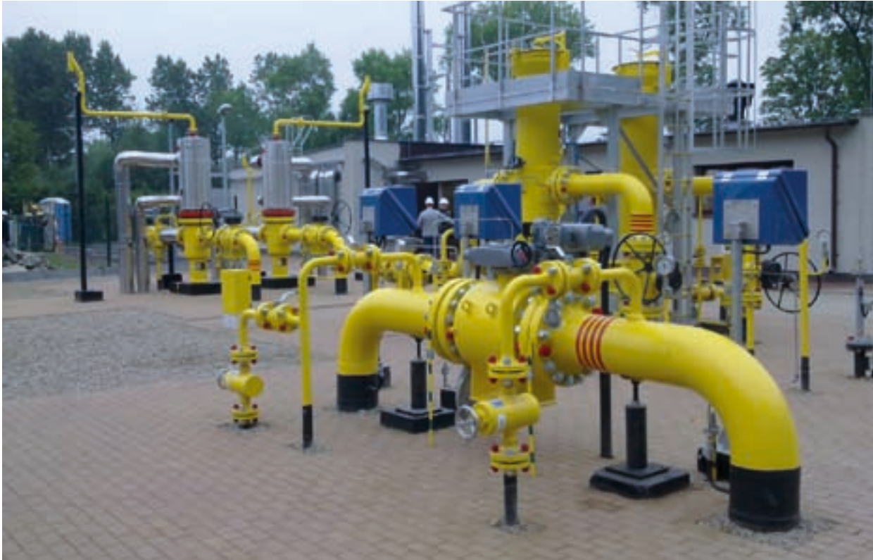
Gas pipeline Wloclawek-Gdynia, the hub in Wiczlino (photo: GAZ-SYSTEM S.A.)
